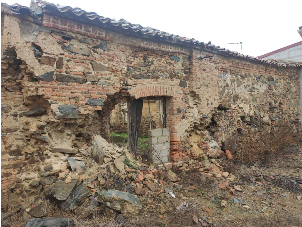
Detail of one of the windows where the original stone-and-brick construction can be observed.
