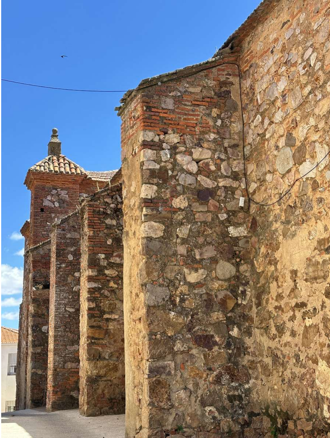
Masonry walls reinforced with granite ashlar blocks at corners and openings. © ARZOBISPADO DE TOLEDO. TOLEDO. ESPAÑA
