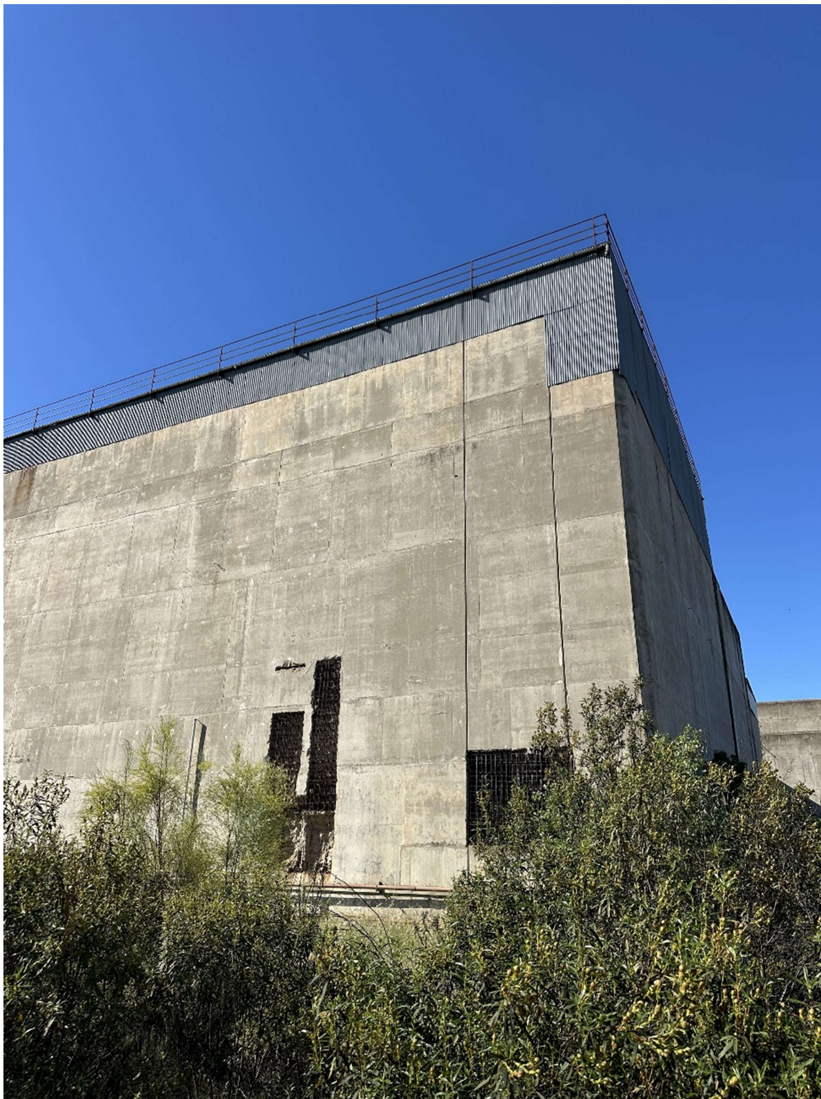
Hollows showing the attempts made to demolish the facilities.
