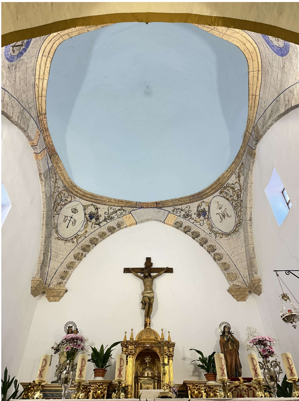
Irregular dome of the Church of Santa María Magdalena. © ARZOBISPADO DE TOLEDO. TOLEDO. ESPAÑA
