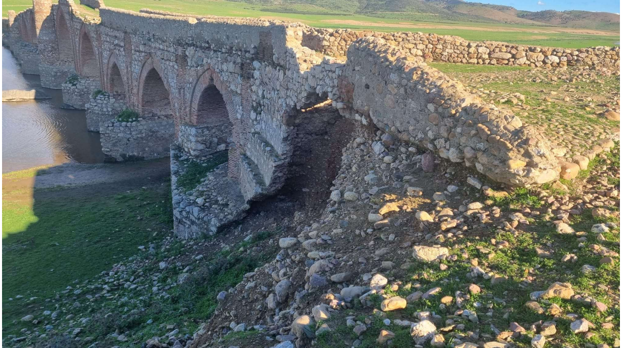
The deterioration of the construction led to its inclusion on the Hispania Nostra Red List in 2022.
