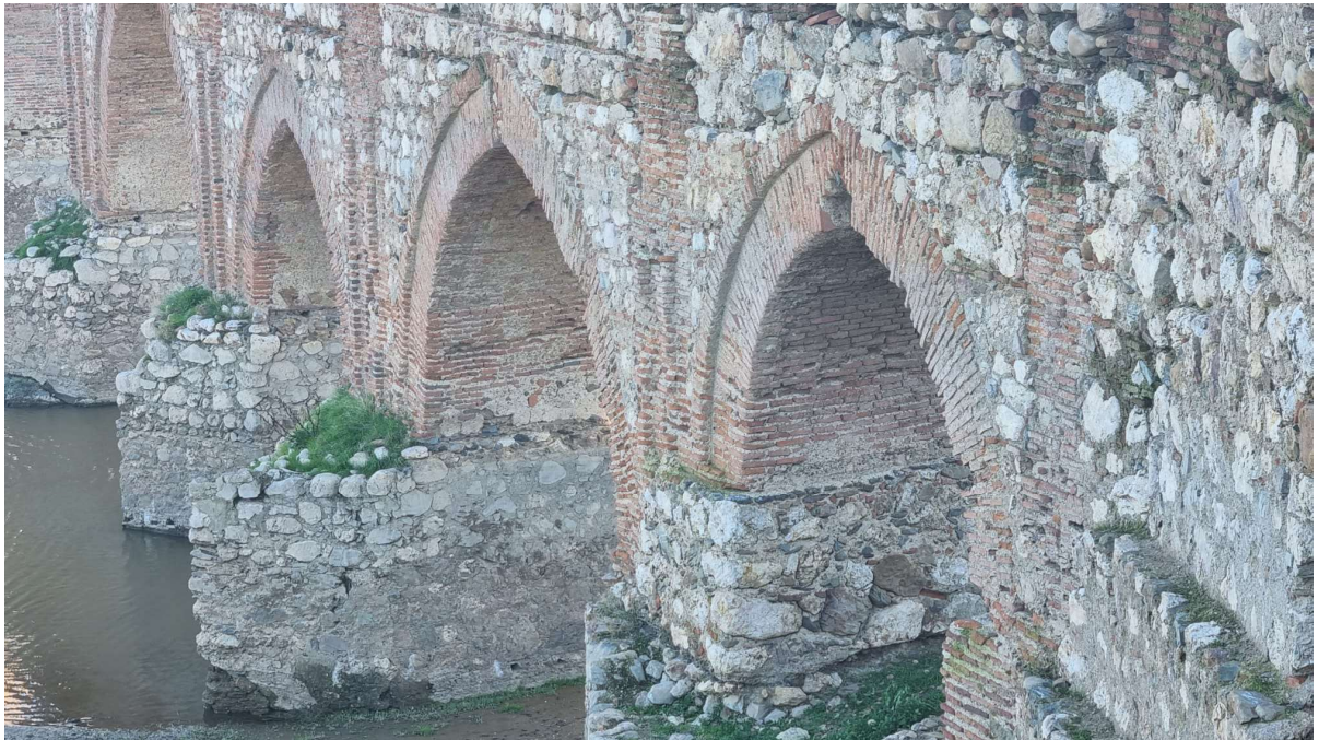
The five southernmost arches maintain a notable stylistic relationship with another four northern arches.
